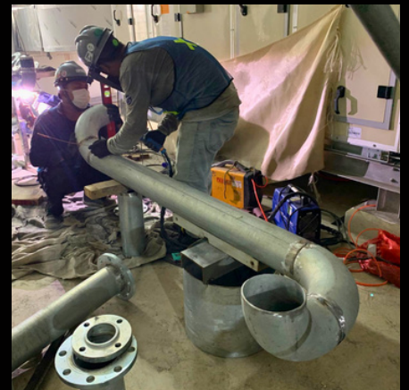
Instalasi Pipa Chiller AHU
