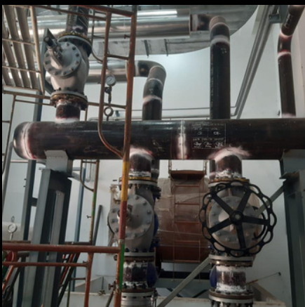
Pipa Hider Boiler
