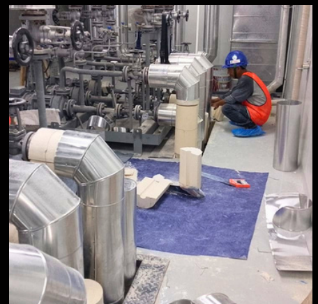
Jacket Insulasi Steam Pipe PT. BANGKIT DJAYA PERKASA
